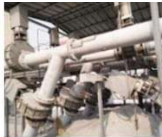
prone to cracks
